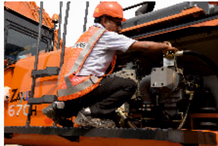
Centralized Filter System
